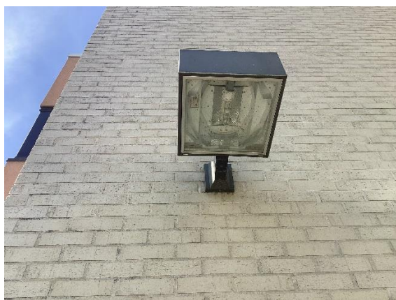
Old Exterior Lighting
