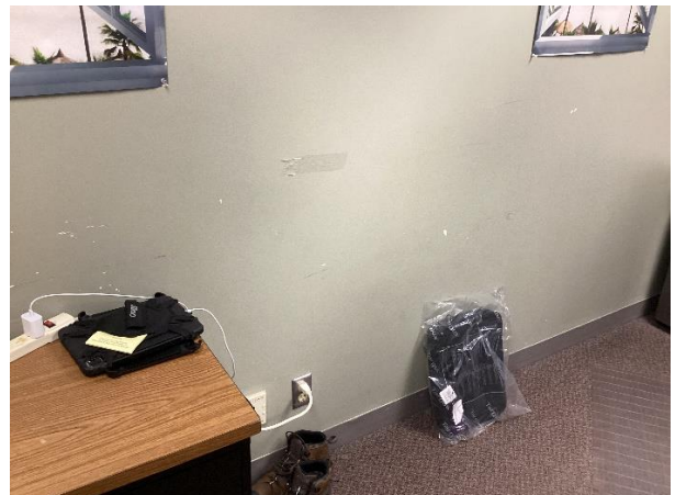
Damaged Wall Surfaces
