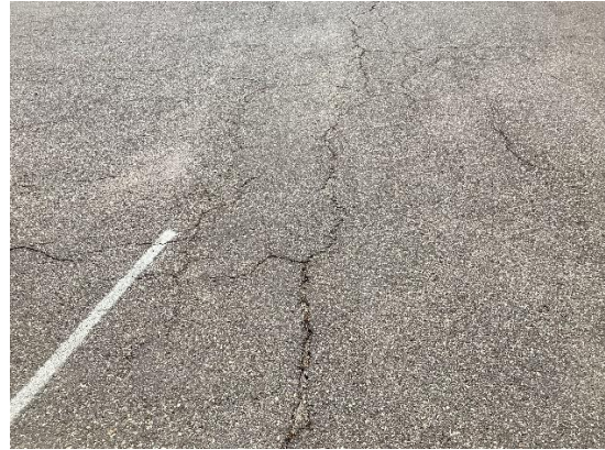
Dry, Cracking Bituminous
