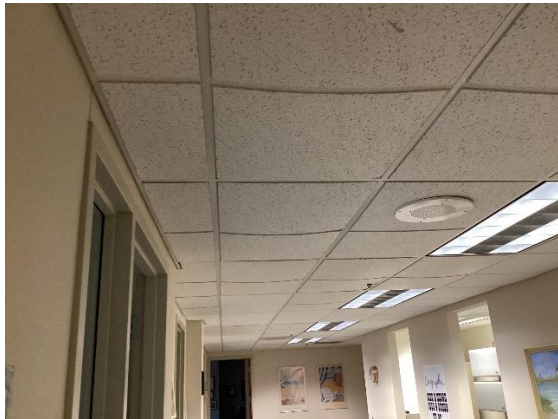
Sagging Ceiling Tiles
