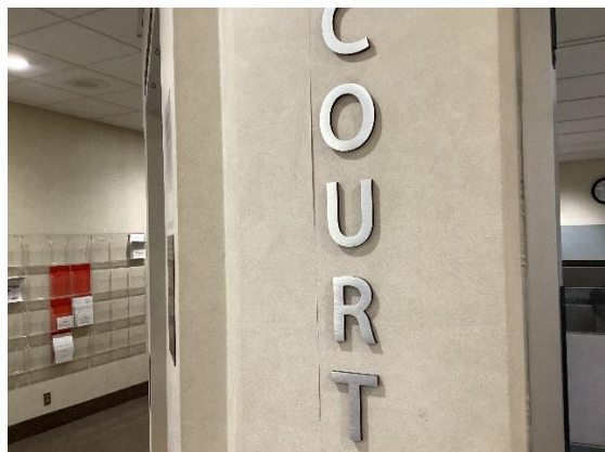
Damaged Wall Covering
