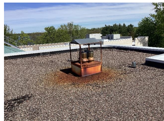
Rusting Boiler Exhaust
