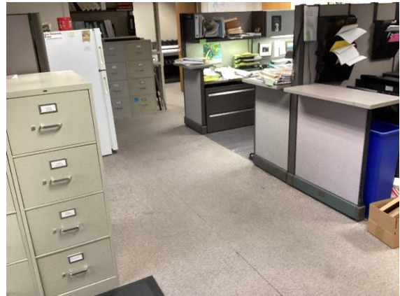
Old Damaged & Stained Carpet
