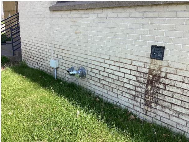
Stained Block and Eroded Mortar
