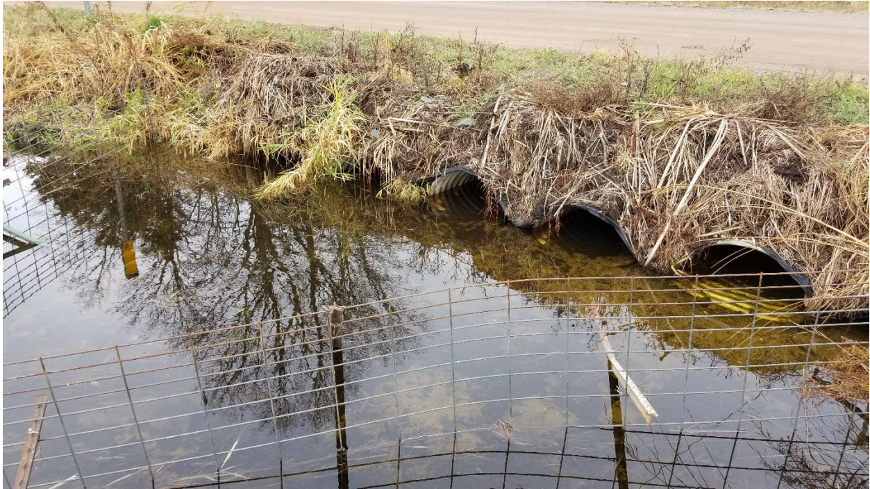
Photo: blockage at the upstream end of outlet pipes at Swamp Lake
