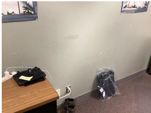
Damaged Wall Surfaces
