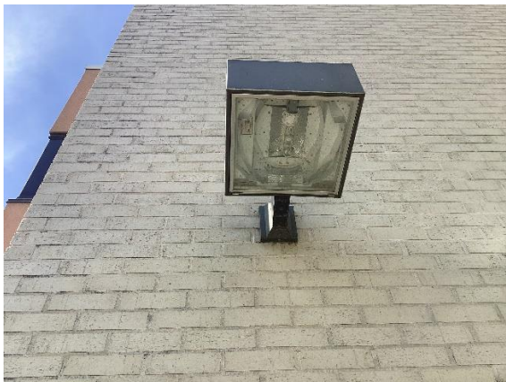
Old Exterior Lighting
