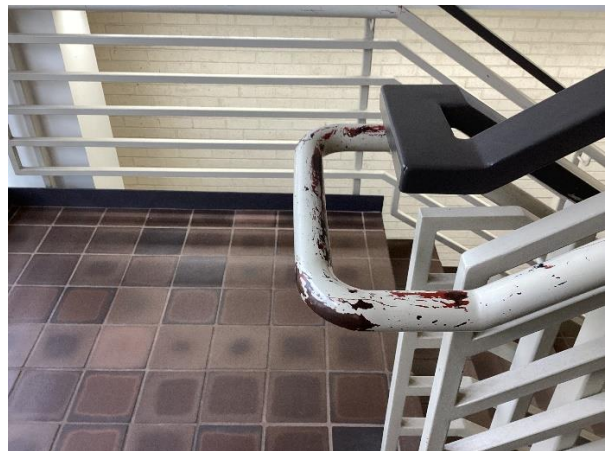
Paint Damage on Handrails
