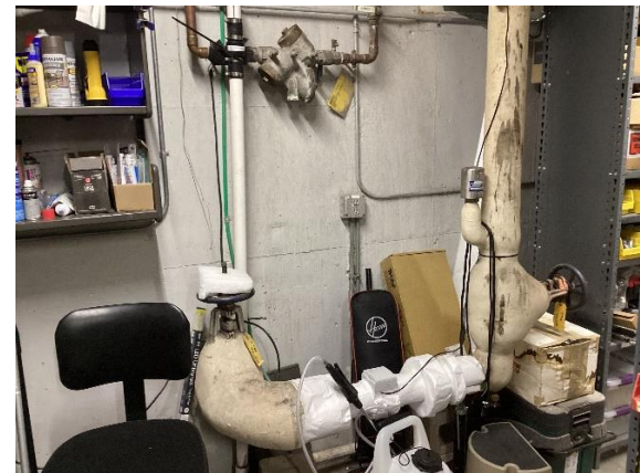
Asbestos Pipe Insulation
