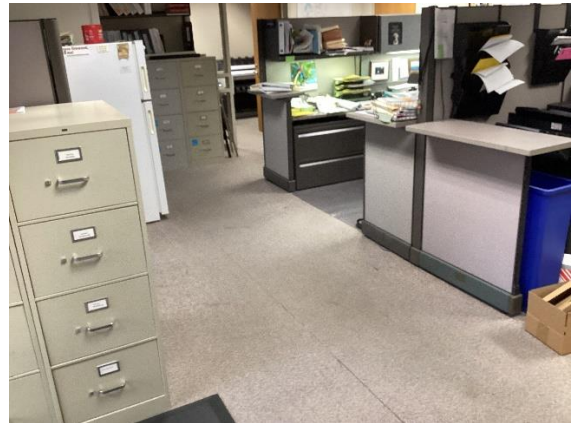
Old Damaged & Stained Carpet
