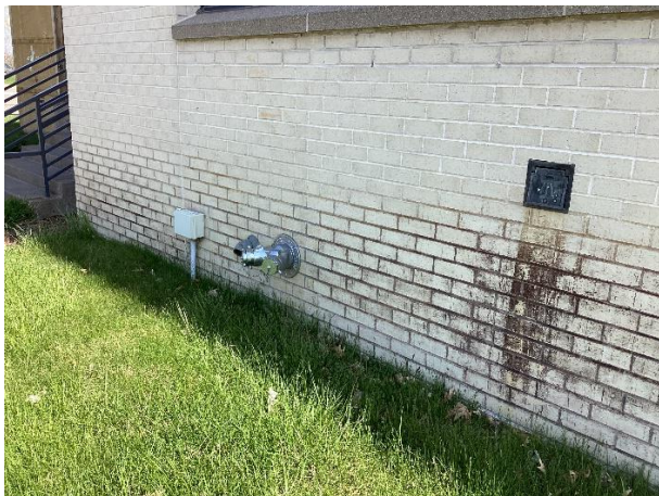
Stained Block and Eroded Mortar
