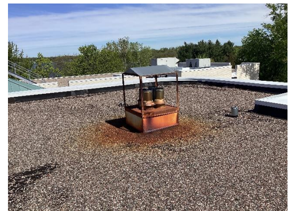
Rusting Boiler Exhaust
