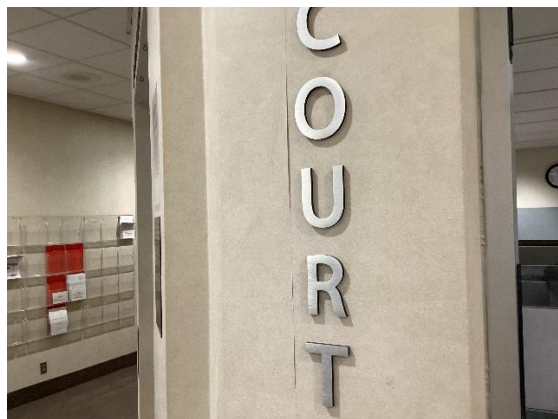
Damaged Wall Covering
