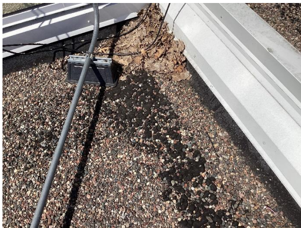
Bubbling on Roof
