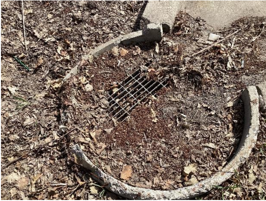
Clogged Parking Lot Area Drain
