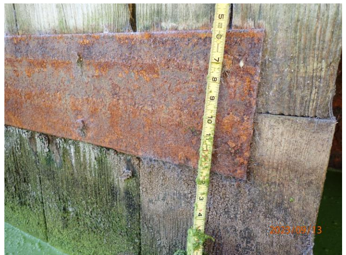
TYPICAL SURFACE CORROSION OF STEEL BANDING
