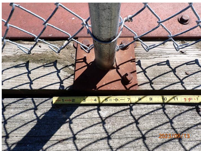
TYPICAL FENCE POST BASE CONDITION
