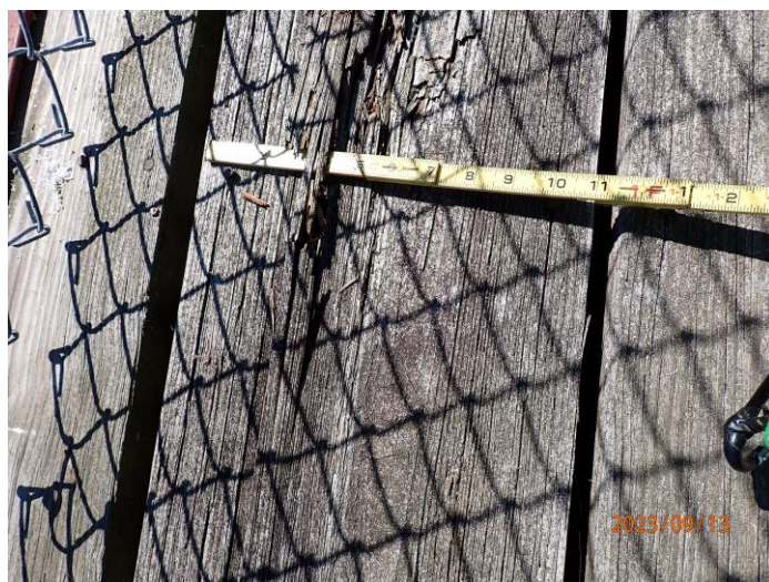
TYPICAL ABRASION OF WEIR DECK
