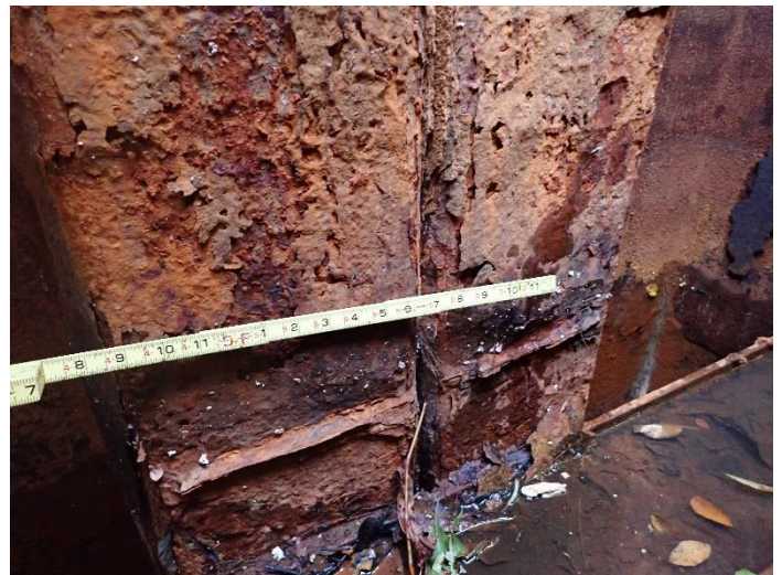
TYPICAL STEEL SHEET PILING CONDITION
