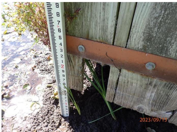
AREA OF MINOR DAMAGE AT SOUTHEAST CORNER OF WEIR LOOKING WEST
