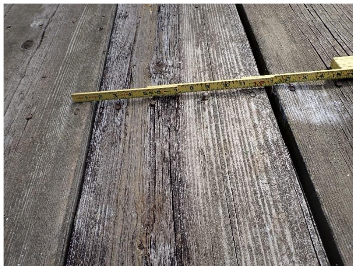
TYPICAL LOOSE NAILS STARTING TO PULL OUT
