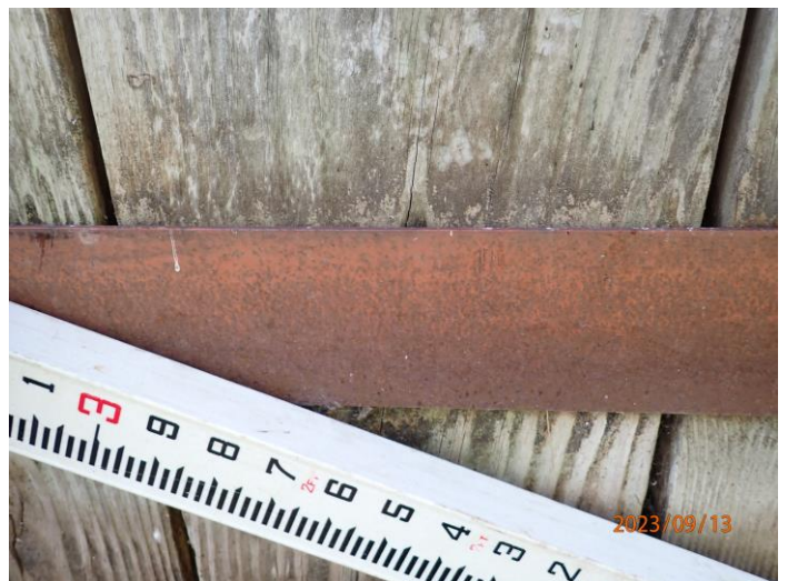
TYPICAL SURFACE CORROSION OF STEEL BANDING
