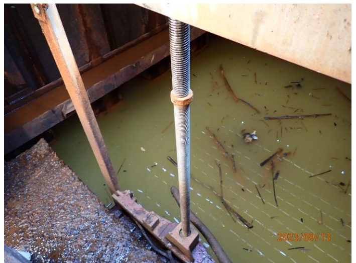
GATE LIFT STAINLESS STEEL THREADING CONDITION
