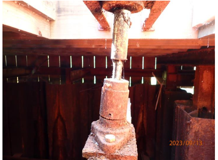
GATE LIFT DISPLACEMENT LOOKING WEST
