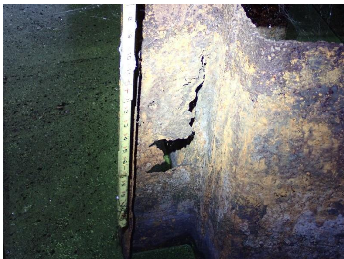
TYPICAL CORROSION HOLE AND SECTION LOSS OF VERTICAL COLUMN WEB
