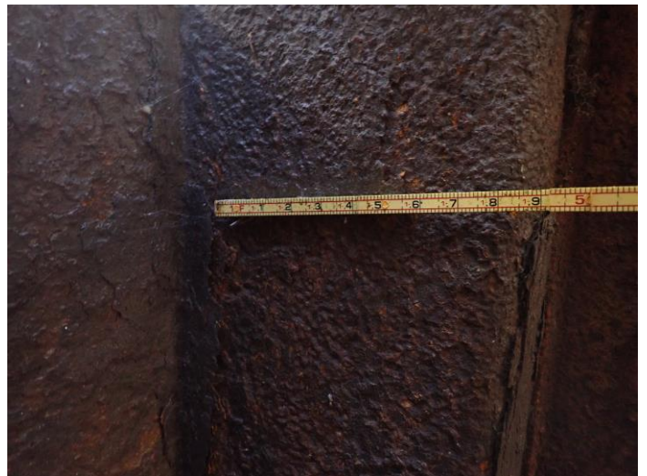
TYPICAL STEEL SHEET PILING CONDITION
