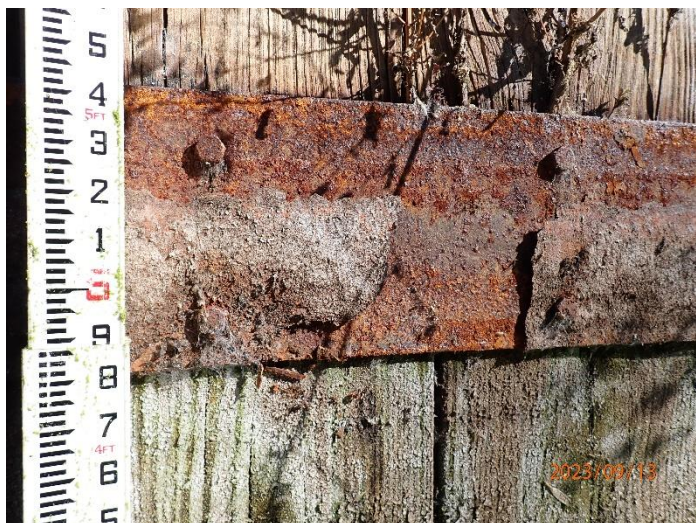
AREA OF ISOLATED SECTION LOSS OF STEEL BANDING AT SOUTH FACE LOOKING NORTH
