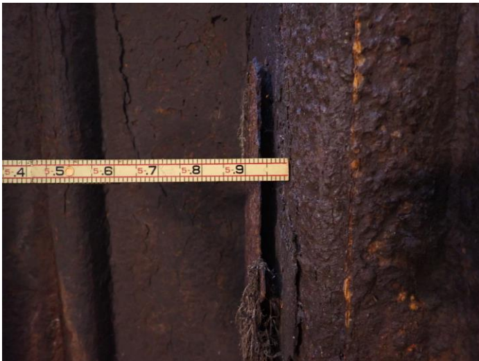
TYPICAL LAMINATED RUST OF STEEL SHEET PILING
