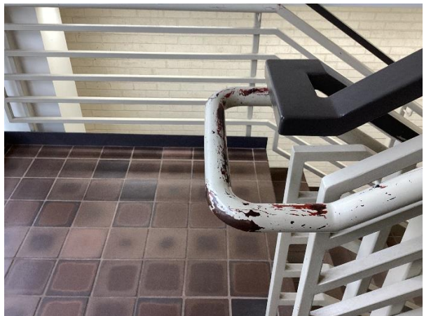
Paint Damage on Handrails
