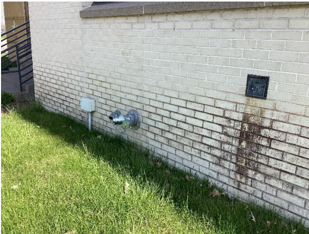
Stained Block and Eroded Mortar
