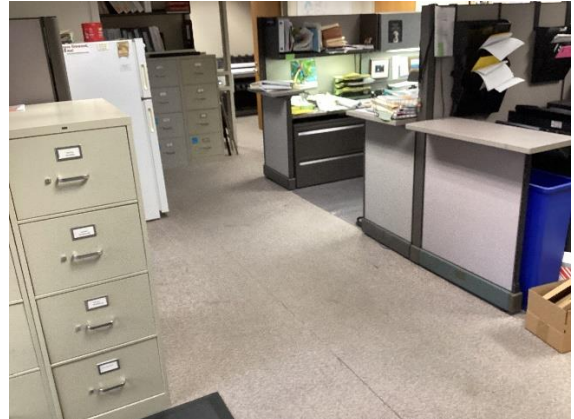
Old Damaged & Stained Carpet
