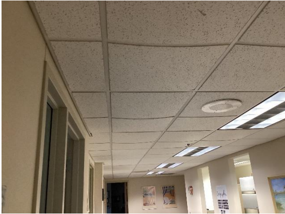
Sagging Ceiling Tiles
