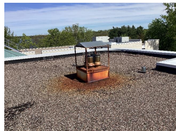
Rusting Boiler Exhaust
