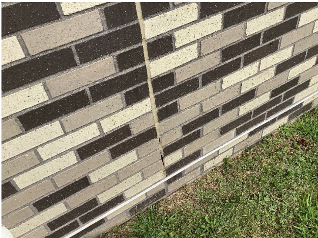
Missing and dry sealant
