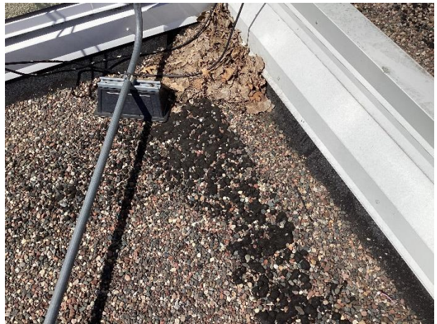
Bubbling on Roof
