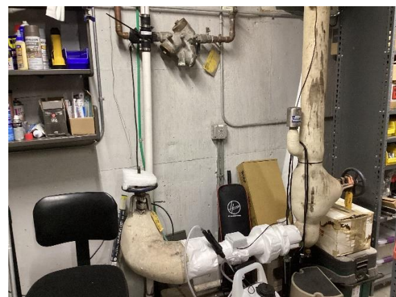
Asbestos Pipe Insulation
