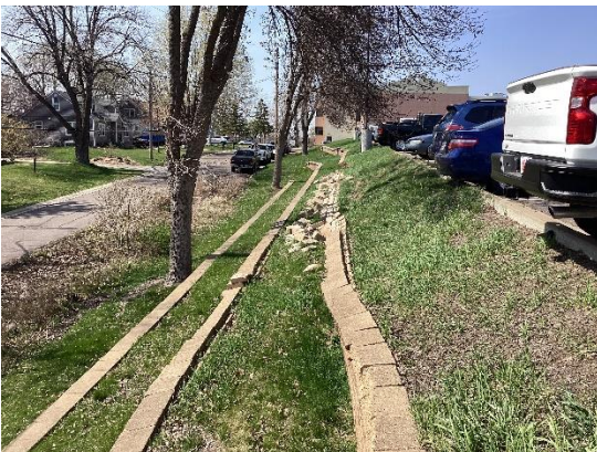
Failing Retaining Walls
