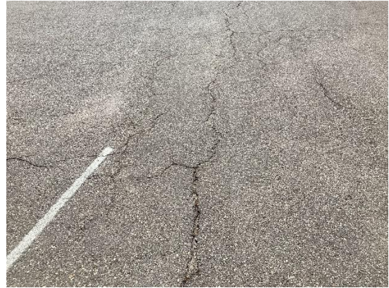
Dry, Cracking Bituminous
