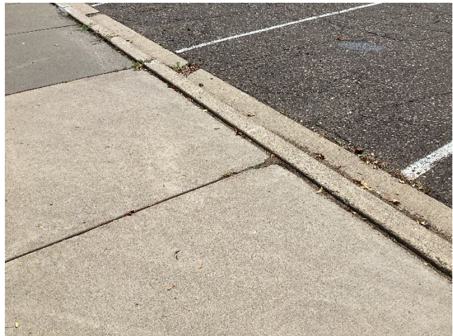
Minor settling of walk
