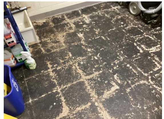
Tiles Removed, Suspect Mastic Exposed
