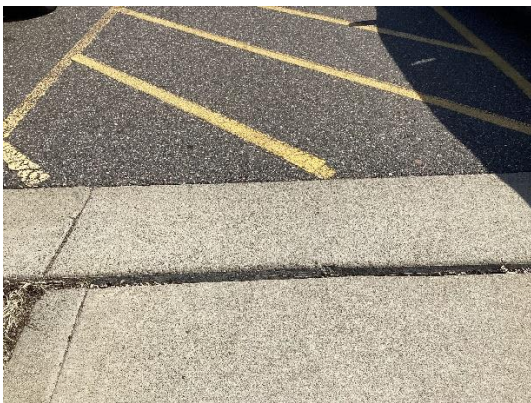
Settled Concrete (Trip Hazard)
