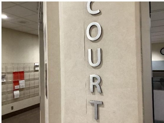
Damaged Wall Covering
